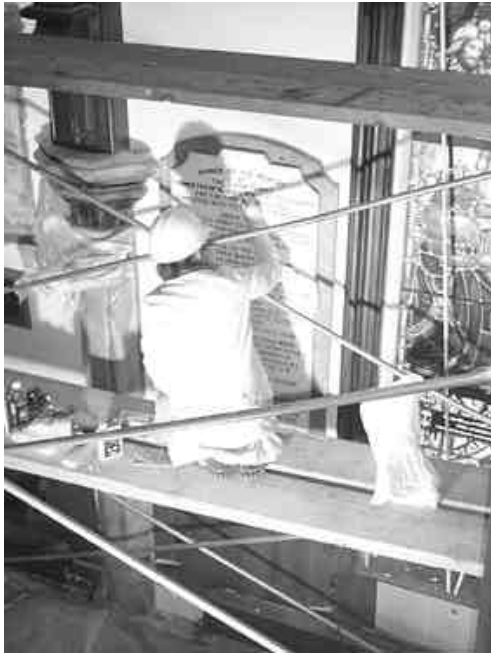
Conservation Specialist, Kellie McIvor is shown restoring one of the wall memorial plaques.
